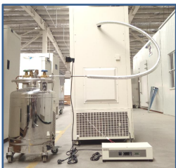
LN 2 /CO 2 backup system
